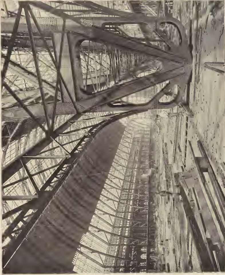
CONSTRUCTION OF THE GREAT MANUFACTURES AND LIBERAL ARTS BUILDING. Interior View, 1864, showing Dome's Truss.
